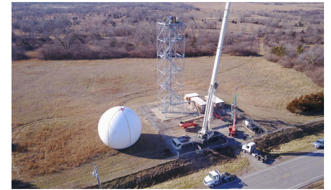
As part of the WSR-88D Service Life Extension Program, the NWS office in Des Moines, IA undergoes a radar pedestal refurbishment.
