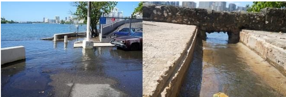
Figure 13. Photos of areas of "nuisance flooding" and storm drainage system in south/southwest portion of lagoon (Photos: PRDNER).
