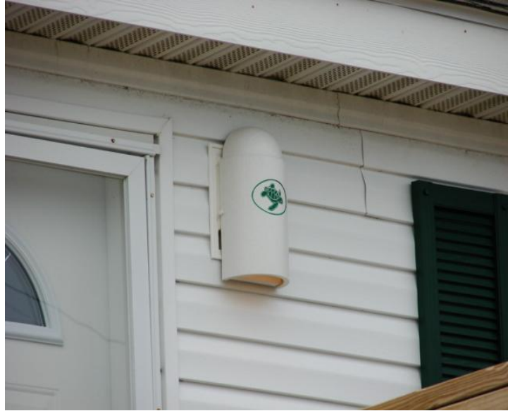
Figure 2. Onslow Beach housing unit showing canister lighting.
