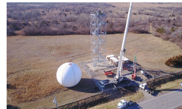
As part of the WSR-88D Service Life Extension Program, the NWS office in Des Moines, IA undergoes a radar pedestal refurbishment.
