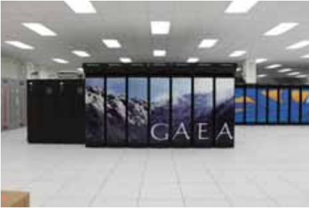
NOAA High Performance Computing Systems at Oak Ridge National Laboratory
