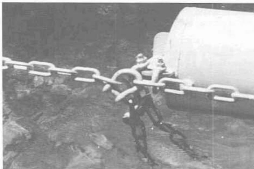
Figure 25. - Photograph of a deformed shackle used to connect the Carr tailrace curtain to a shore anchor.
