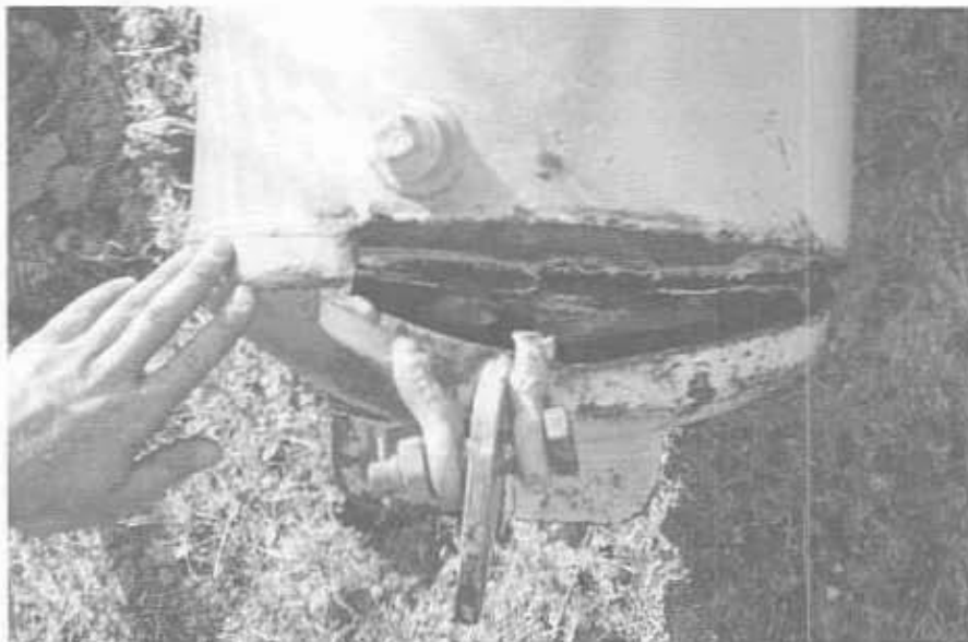
Figure 24. - Photograph of a failed weld on a Carr tailrace curtain top boom floating tank.
