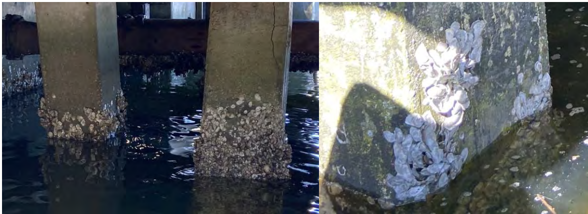
Figure 26. Evidence of oyster growth at Pier Romeo
