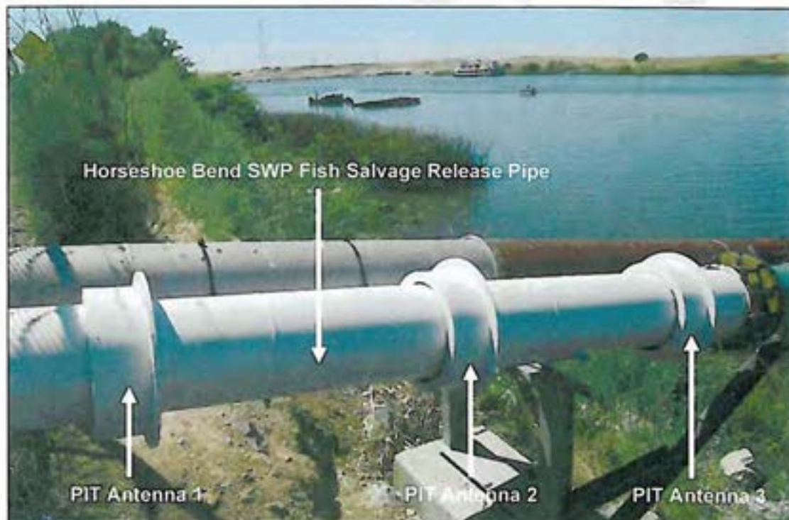
Figure 37. PIT antennas installed around the release pipe at the Horseshoe Bend, SFPF salvage release site.
