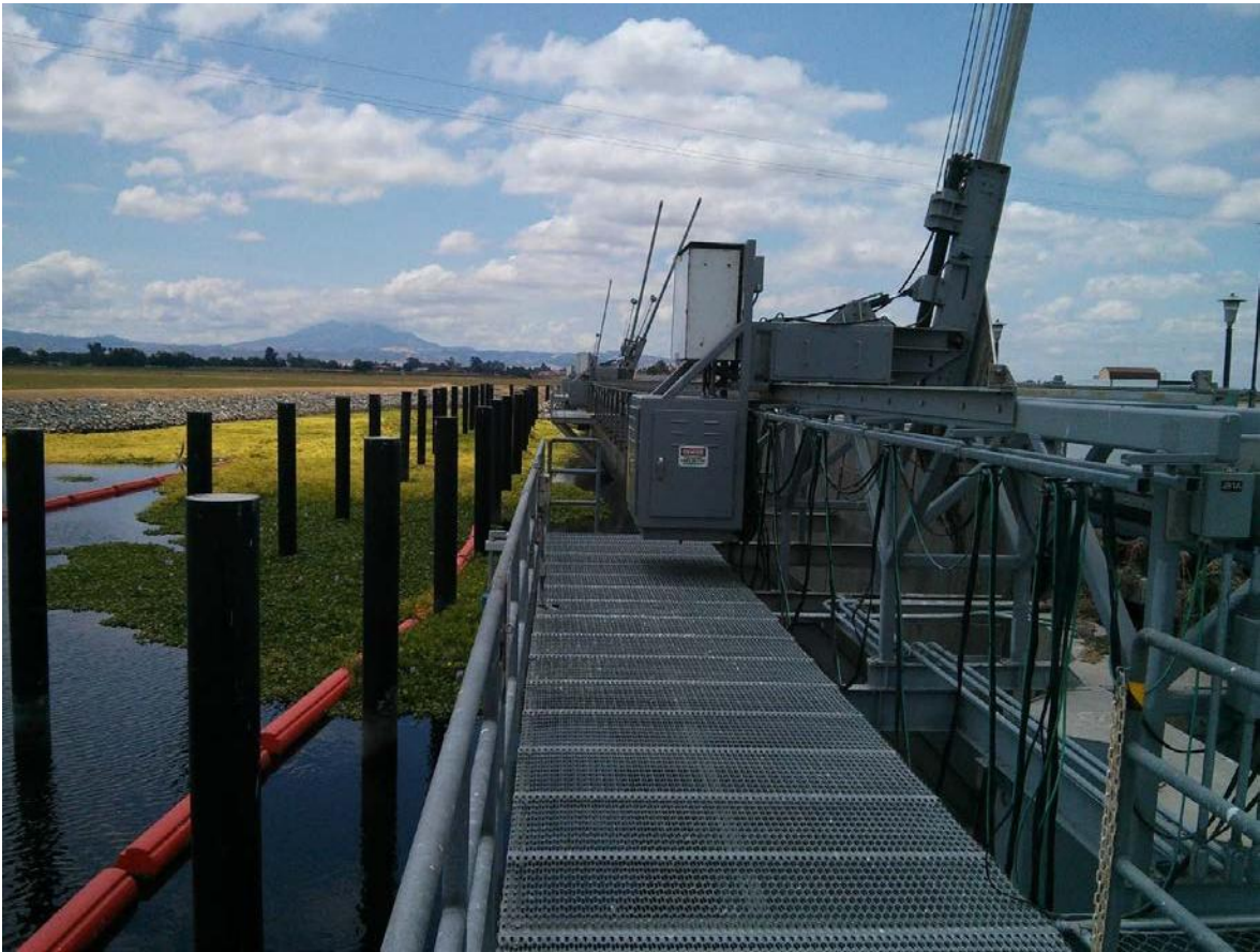
Figure 5. Existing safety deck and hydraulic rakes on the northeast side of the RSFS (Reclamation 2016).
