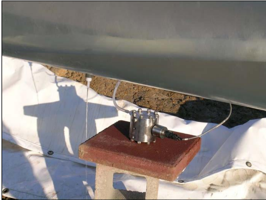
Figure 6- Close-up view of one of the pressure transducers installed to measure flow in the release pipe.
