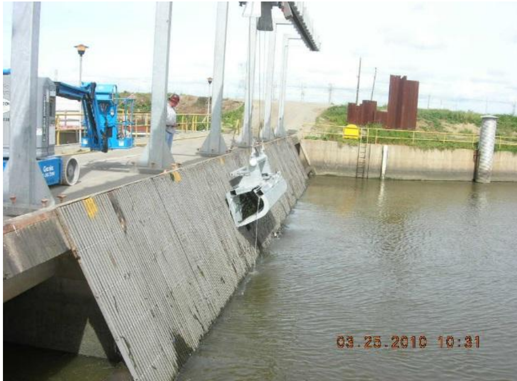
Figure H-1. Photograph of trash rack with 2 panels removed in spring 2010 (arrows indicate removed panels).
