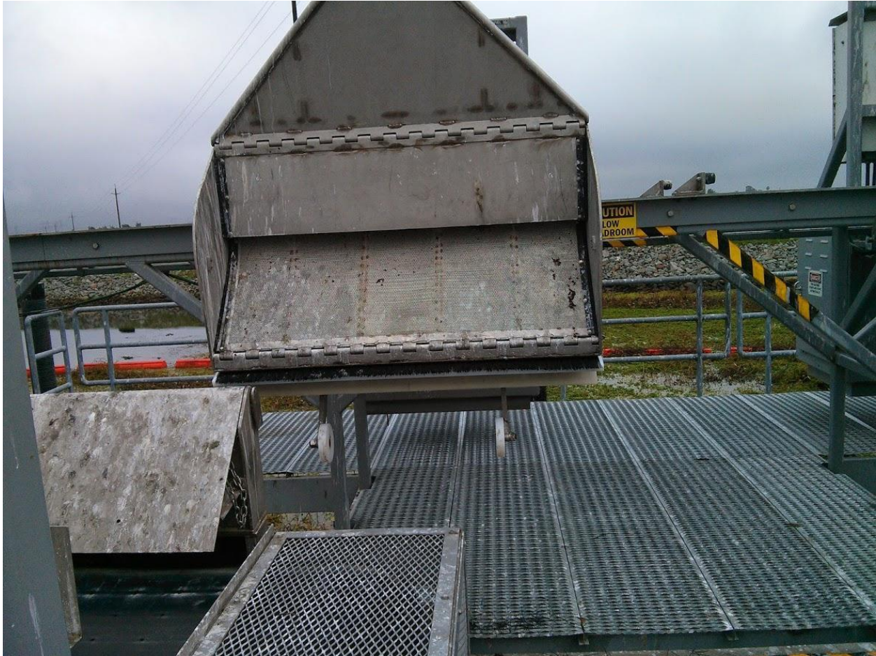
Figure 4 Prototype Rake Installed in 2015 at Rake Number 2
