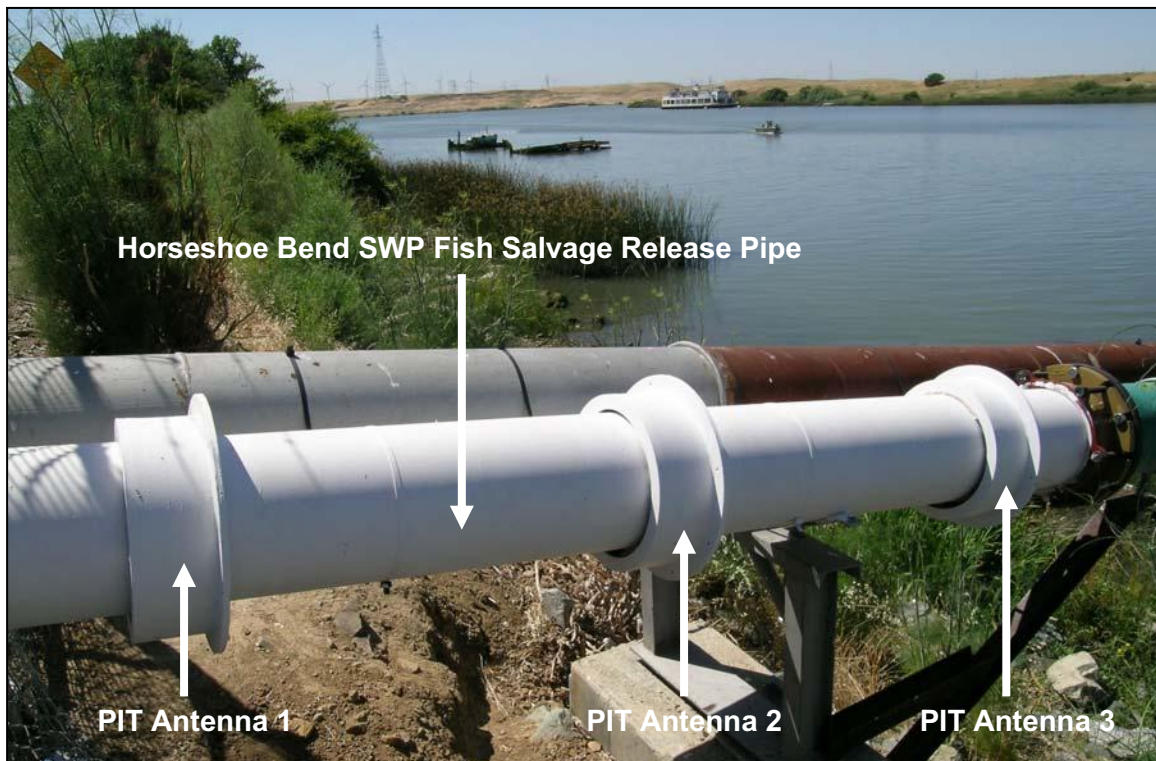
Figure 37. PIT antennae installed around the release pipe at the Horseshoe Bend, SFPF salvage release site.
