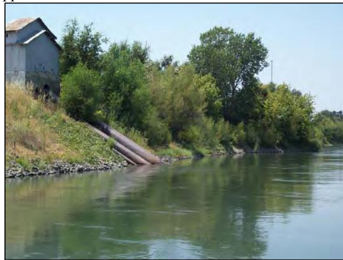
Appendix Figure 51. The Alamo pump intakes looking in an upstream direction.
