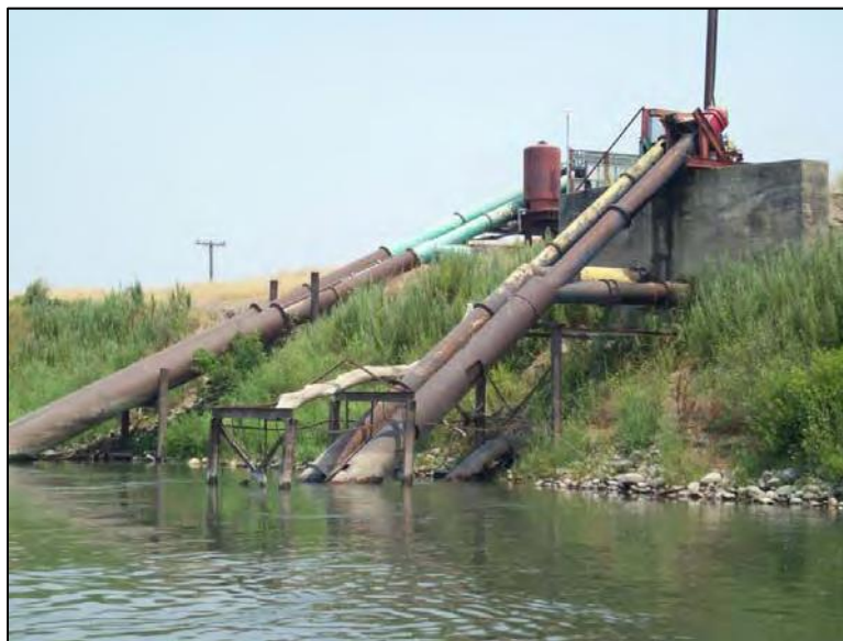
Appendix Figure 72. The Cranmore pump intakes (foreground) looking in an upstream direction.
