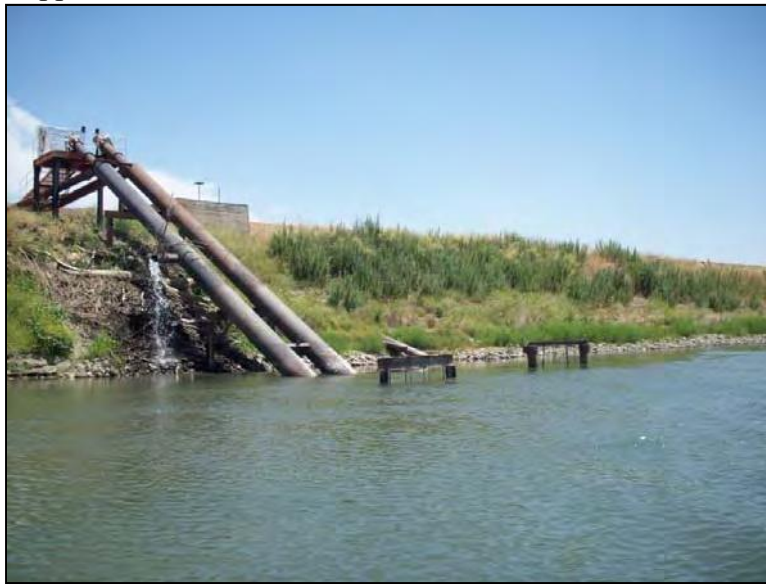
Appendix Figure 30. The Oji pump station intakes looking in a downstream direction.
