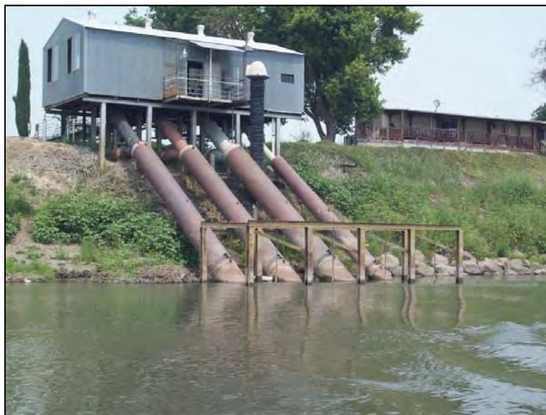
Appendix Figure 16. The State Ranch pump station intakes looking in a downstream direction.
