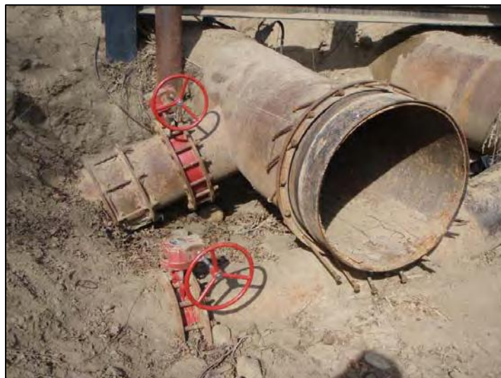
Figure 119. Flow bypass valves (red) at the Sycamore diversion. The two large-diameter pipes on the right lead to the Sycamore canal through a levee. Each pipe has a separate flow bypass valve on the left that can be used to route excess pumped flow back to the Sacramento River. The left intake pipe is disconnected for pump maintenance.
