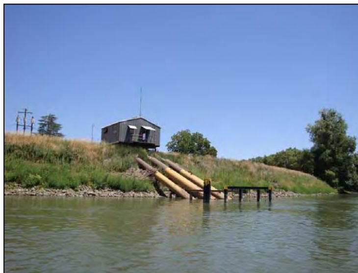
Appendix Figure 44. The Portuguese Bend pump station intakes looking in a downstream direction.
