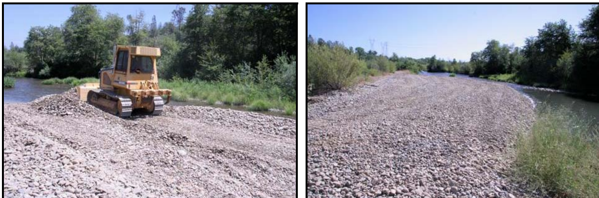
Figure 20. Downstream views of the lower lateral berm above Phase 3A during and following construction in July 2010.
