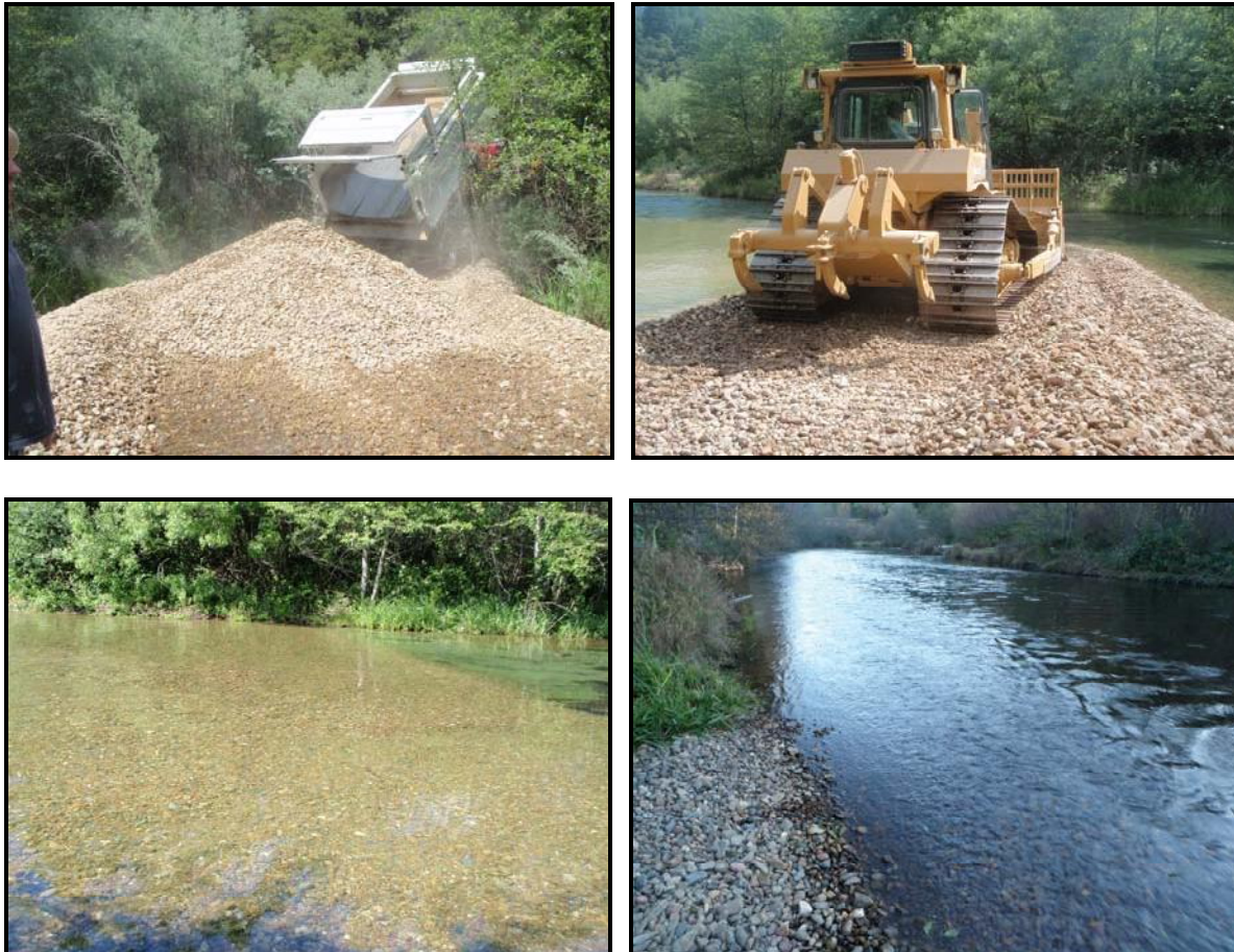
Figure 11. Gravel injection above NEED Camp Bridge occurring through a gap in the left bank vegetation. The 2009 as-built injection showing the upstream end and a November 2010 view downstream showing the increased water surface slope through the pool.
